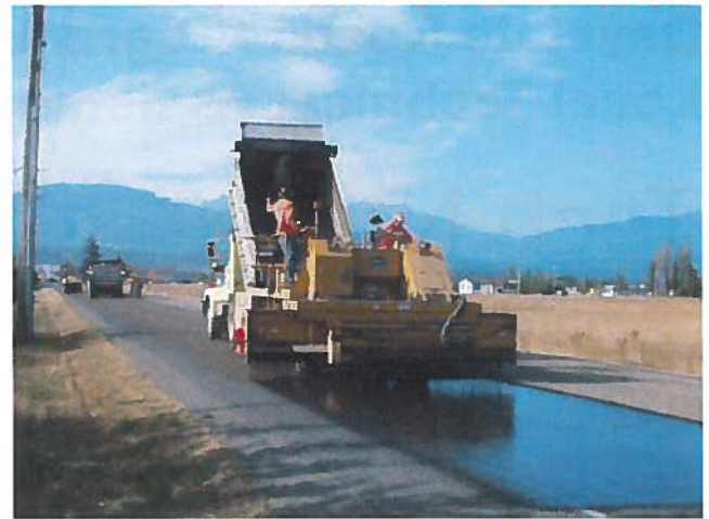
5/8" and smaller crushed rock chips are applied to the liquid asphalt with a chip spreading machine
